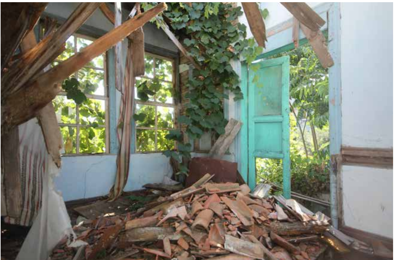
Fig. 3: Second floor's sofa and the timber door opening to non-existent room on the west
