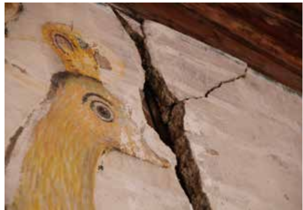
Fig.15: Large crack on the south wall
