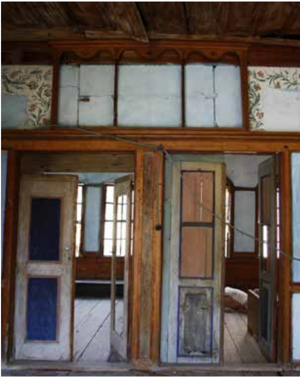
Fig.7: Doors opening to the rooms to the east of the sofa and the iconostasion on top
