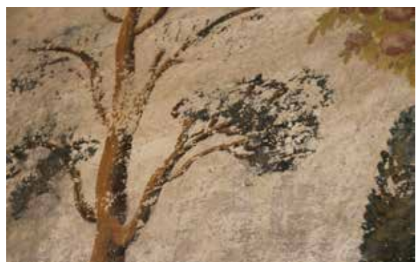
Fig.17: Loss of paint on the south wall of the northwest room
