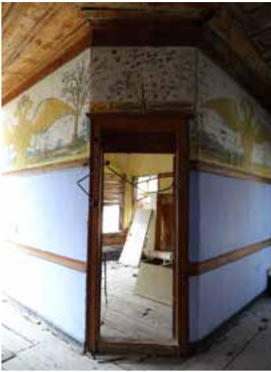
Fig.5: General view of the northern and western wings of the sofa (inner hall) and northwest room
