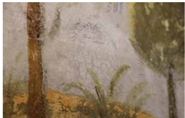
Fig.16: Deterioration of the paint layer on the east wall
